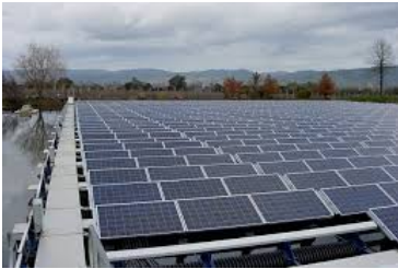
A typical solar installation. A presentation on Solar Power was given at the Annual Meeting
